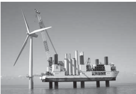
Figure 2 Lynn and Inner Dowsing wind farms under construction. Image courtesy of Centrica.
