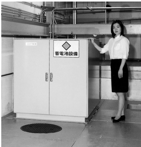
Photo 4. 50-kW system for office buildings
