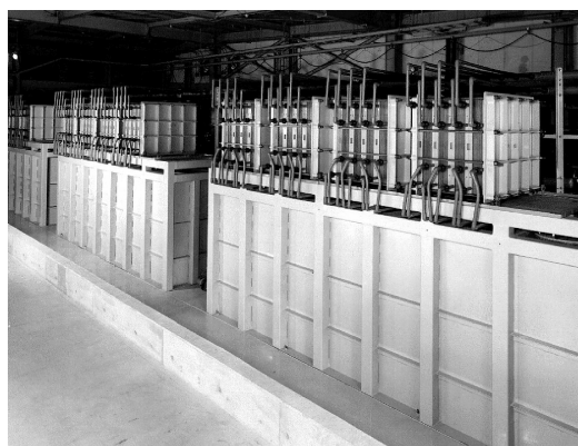
Photo 1. 450-kW battery system in operation
