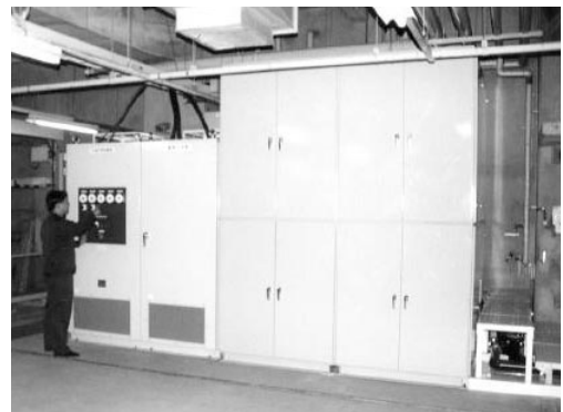
Photo 5. 100-kW system installed in an office building
