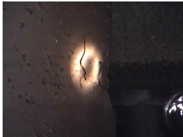
Exhibit 8-6. Fatigue due to cyclic loading caused cracks and spalling in concrete.
