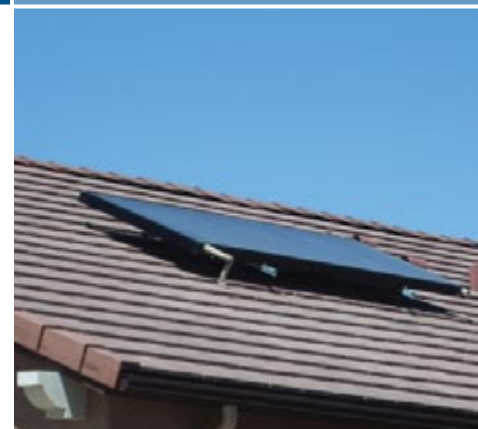
With help from Building America research, Pulte selected closed-loop, active solar water heating units.
