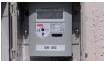
Solar thermal meter used by Lakeland Electric. Photo courtesy of Jeff Curry of Lakeland Electric.
