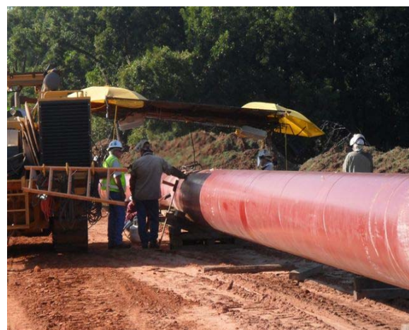
Figure ES-2 36-Inch-Diameter Crude Oil Pipe
