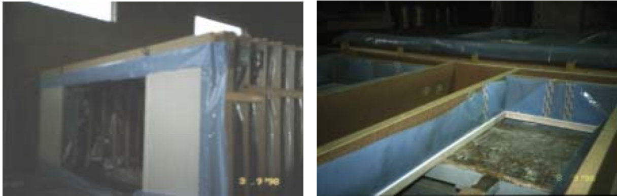
Figure 30 (left): Facade element window opening. The airtight foil joints are carefully glued, the overhanging foil is there to allow for an airtight seal with the next elements
