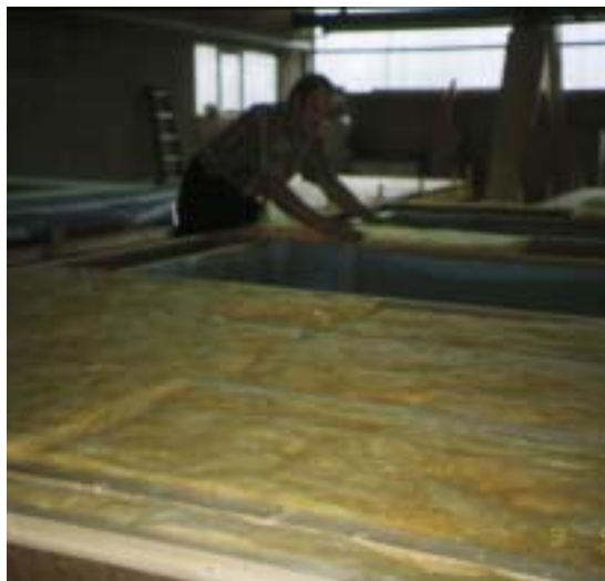
Figure 29: The insulation must lie loose and slightly inflated within the element, so that no cavities are formed later
