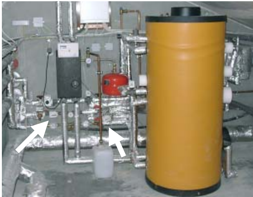
Figure 41: Installation wall on the building services floor with water storage tank. The two heat quantity meters are marked with arrows.
