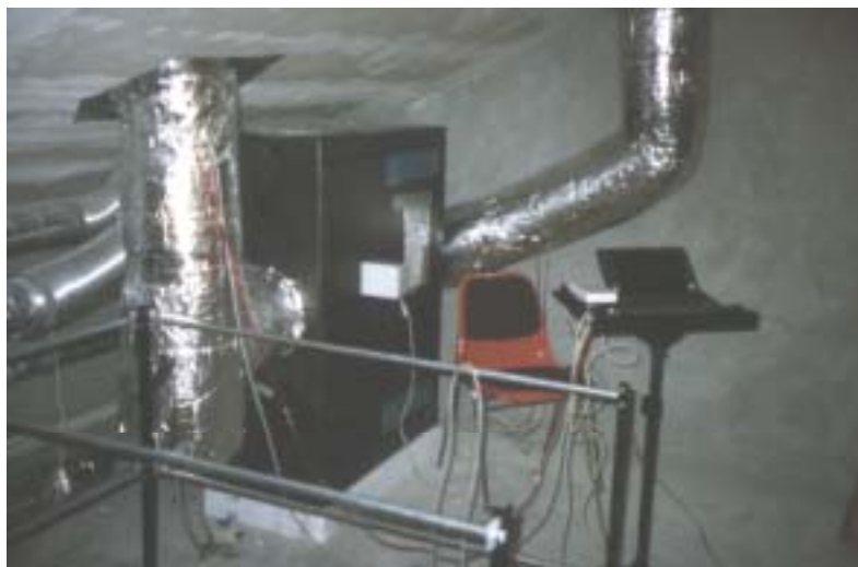
Figure 36: Measurement technology set-up for the balance calibration of the heat recovery system in the building services floor of one of the Passive Houses. With the use of pressure measurement, the volume flows at the differential pressure sensors in the in- (right) and outflow (left) ducts were determined and evaluated. The outputs of both ventilators were individually set-up with the manufacturer's operating device.
