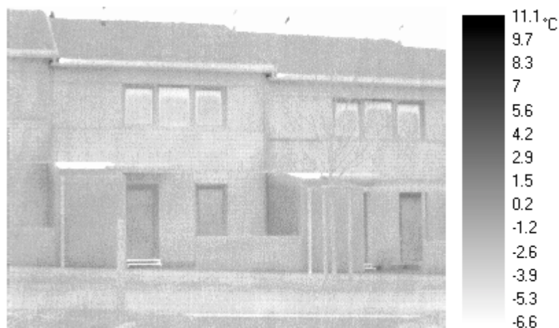
Figure 34: Outdoor thermograph of a section of the houses in row 9 (north side). The area under the roof overhang and under the canopy over the main door seem warmer, since these areas are „covered“ from radiation into the cold night sky. Otherwise, the facades show continuous low temperature of around -4\text{ °C} .
