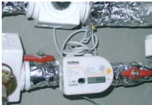
Figure 42: Total heat quantity meter on the installation wall of the building services floor. The cable leads to the temperature sensor (Pt 500) in the supply pipe.
