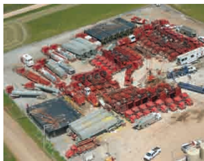
Fig. 5 —Hydraulic fracturing treatment, Woodford Shale, Canadian County, Oklahoma, for which Halliburton provided 52,000 hhp.
