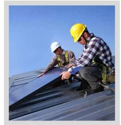
Workers mount PV modules on a private home. These modules use sunlight to generate clean, pollution-free electricity and can reduce or eliminate monthly electricity bills.
