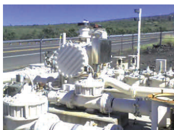
Hawaii County Dept. of Water Supply’s 45-kW in-line hydro plan in Kona
