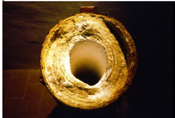
Figure 6 : Scaling in Geothermal pipeline (Bloomquist, 2006)
