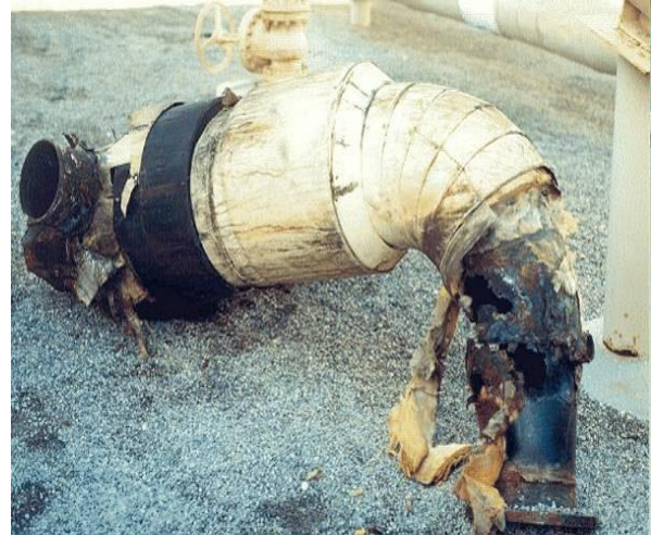
Figure 9: Corroded Steam Vent (Kagel A., 2008)
