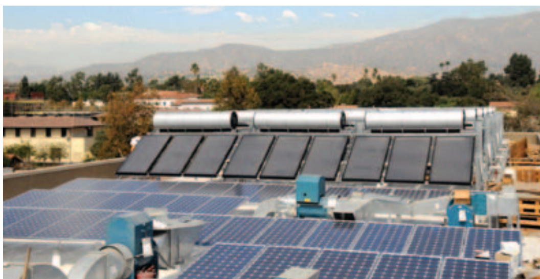
Photo 4.7 An installation of solar PV and thermal collectors on the same roof
