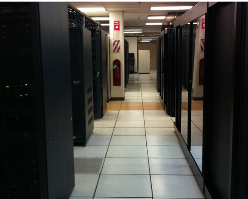
Photo: Data center end-aisle isolation
