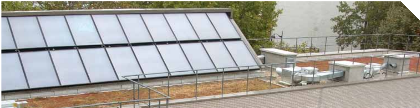
Solar roofing, 19 th
