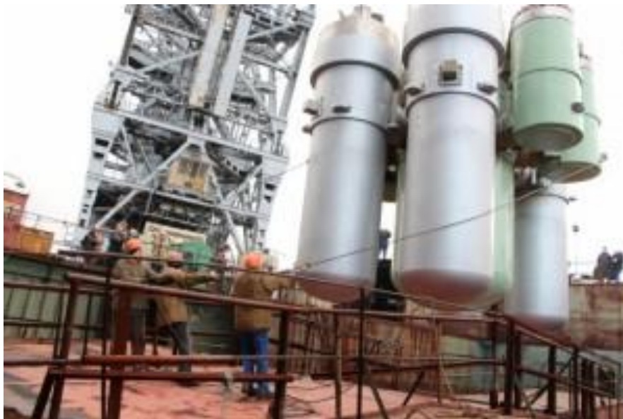
Figure 2. Installation of the Akademik Lomonosov's nuclear reactors in the Baltic Shipyard (available at: http://bellona.org/news/nuclear-issues/nuclear-russia/2015-04-arctic-hopping-russian-deputy-minister-promises-russias-floating-nuclear-plant-next-year ).
