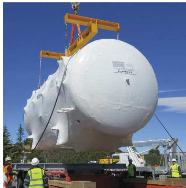
In the basement of the ITER Tritium Plant, six storage tanks will handle the water involved in the tritium recycling process. Europe delivers all six during the year.
