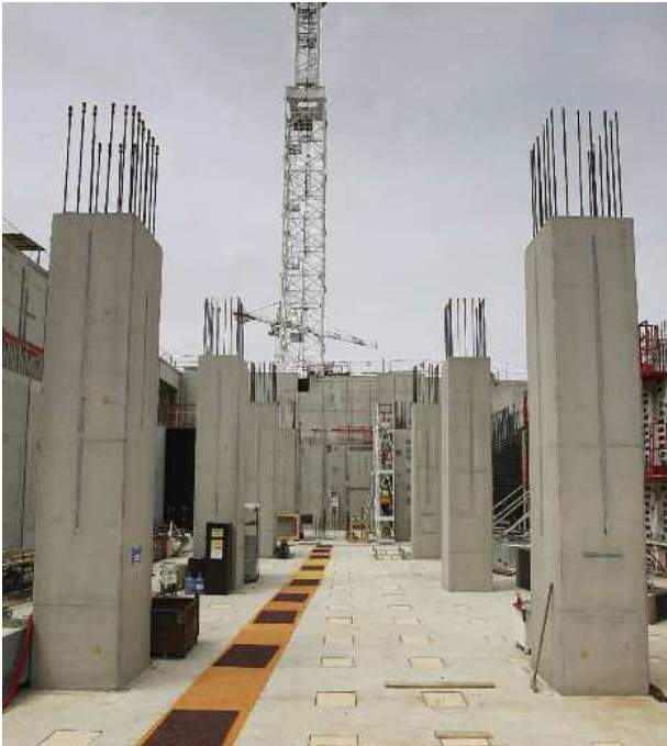
Regular columns in place at the B2-level of the Diagnostics Building will support the next level of construction. Work is also underway on the internal and external walls. Photo: F4E
