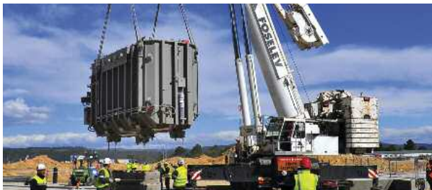
In May the first plant component – an electrical transformer – is installed in its permanent position on site.
