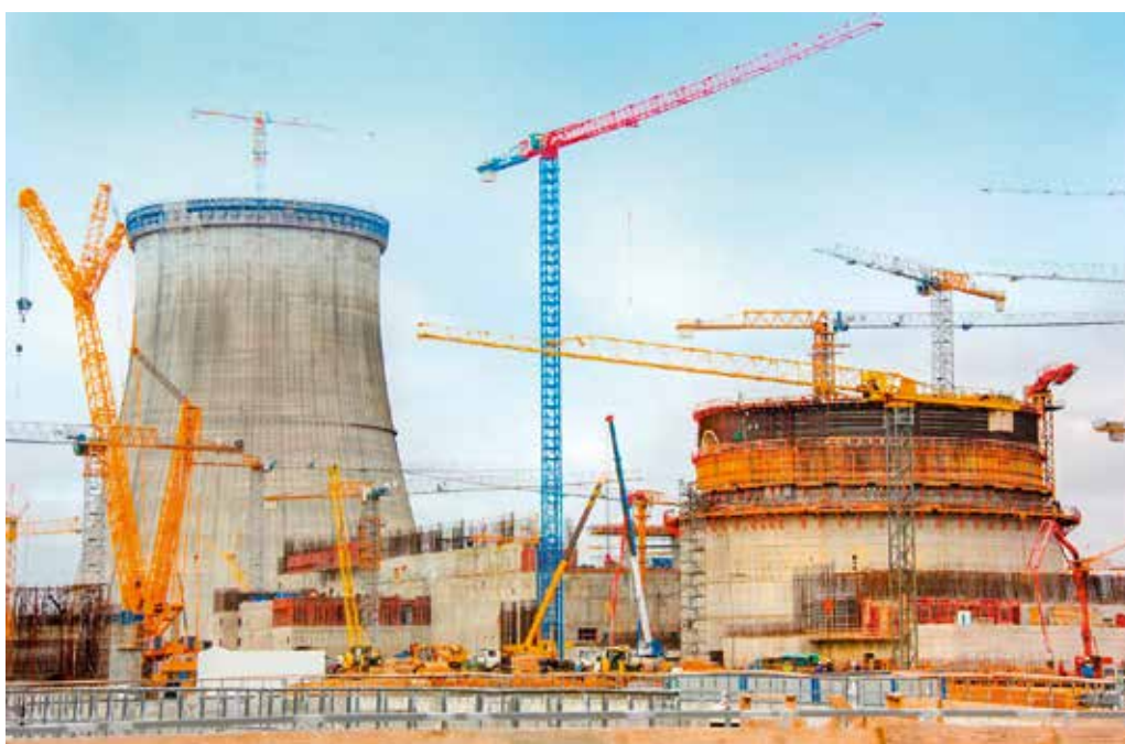
FIG. 1. Construction of Units 1 and 2 of the Ostrovets nuclear power plant in Belarus. (Photograph courtesy of the Directorate for Nuclear Power Plant Construction, Belarus.)
