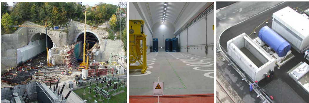
Figure 6. Storage tunnels under construction (left) and with the first casks emplaced (center) at the Neckarwestheim nuclear power plant in Germany, where there was not enough space for a new building. The image on the right shows temporary protection for German storage casks pending construction of a permanent storage building. Sources: Wolfgang Heni and Gesellschaft für Nuklear-Service mbH (GNS). 63
