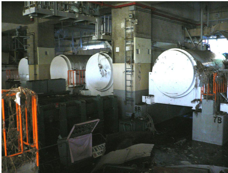
Figure 5. Spent fuel storage casks at the Fukushima Daiichi nuclear power plant after the tsunami had washed through the building. Each cask is 5.6 meters long with a diameter of 2.2-2.4 meters, weighs about 100 tons and contains 6.3 or 8.8 tons of spent fuel. They are designed for spent fuel that has cooled for 5 to 7 years in a pool. Source: TEPCO. 59
