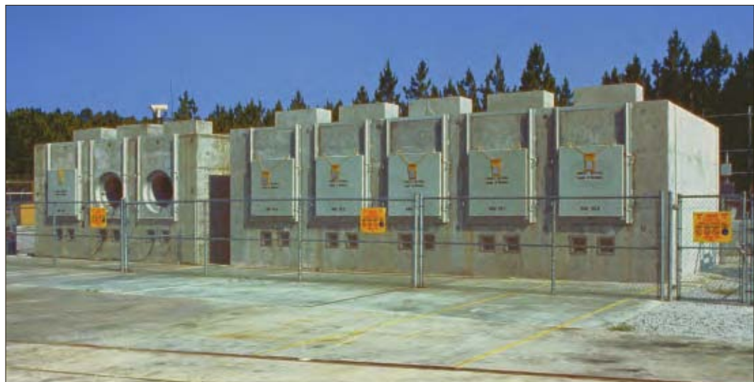
Figure 4.3 Independent Spent Fuel Installation - Dry Cask Storage
