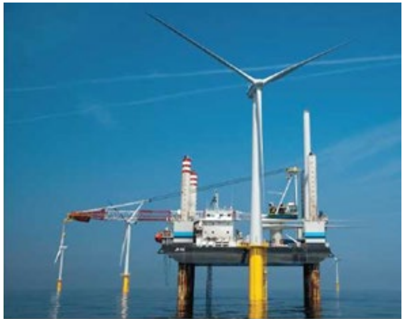
Figure 2. Nobelwind wind farm located in the Belwind concession area in the North Sea approximately 47 km from shore (Source: Nobelwind, http://nobelwind.eu/ )
