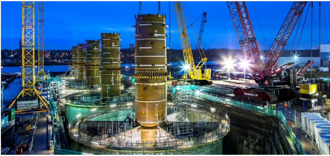
Figure 14. The five “Float-and-sink” gravity based foundations for the Blyth Offshore Demonstration project being manufactured at a dry dock in Newcastle (ORE Catapult, United Kingdom)
