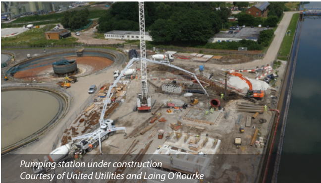
New inlet works under construction Courtesy of United Utilities and Laing O'Rourke
