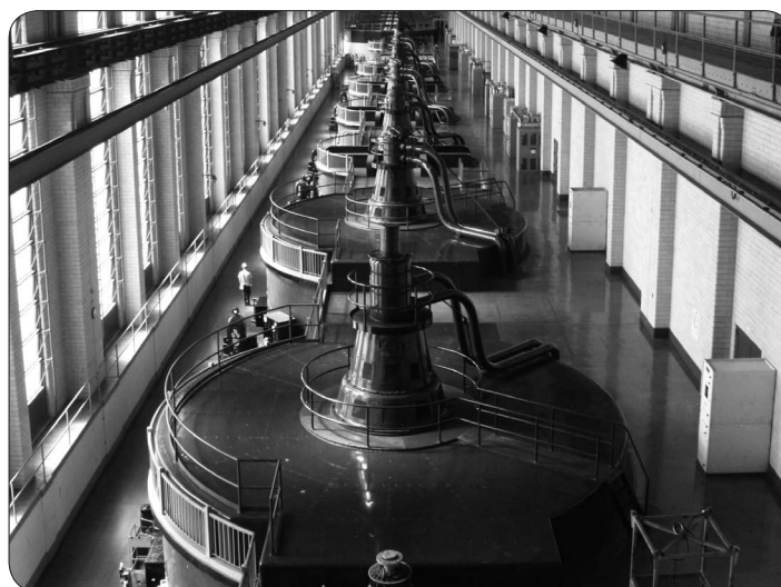
Generators at a hydropower plant.
