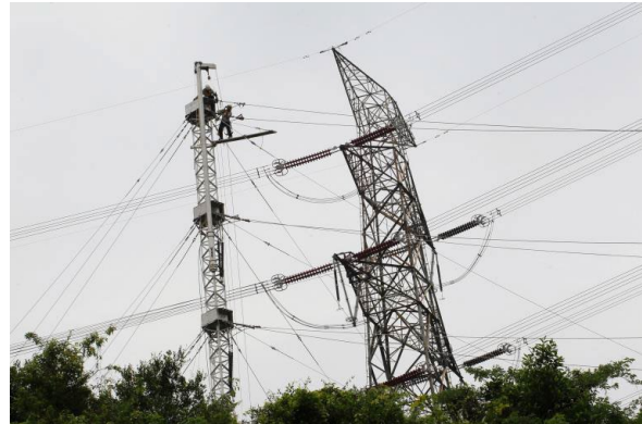
Linesmen are connecting conductors on a 70-foot high temporary mast. The construction of a temporary mast takes a little over 10 days, which is 10 times faster than repairing a damaged tower.
