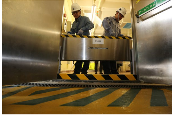
Flood gates are installed at flood-prone transmission substations and distribution.
