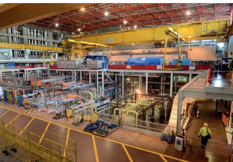
Heysham II turbine hall: Image EDF Energy
