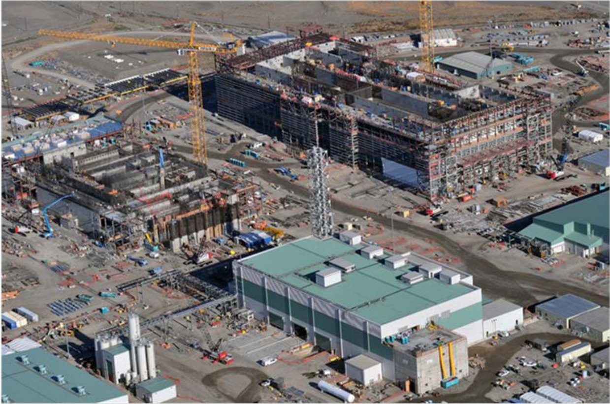
Figure 5-2. Aerial Photo of Waste Treatment and Immobilization Plant from the Southeast (August 2011)
