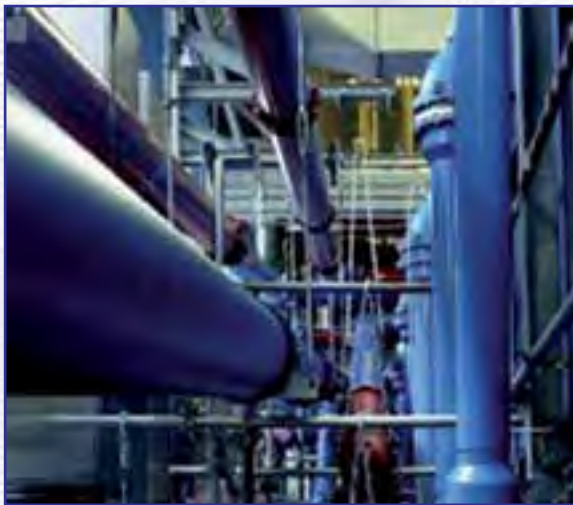
Figure 12: ICRH transmission lines (Photo: J.Polverini and L. Antalova)
