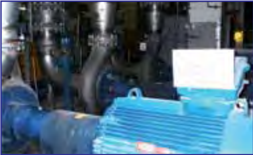
Figure 5: Toroidal field coils cooling pumps
