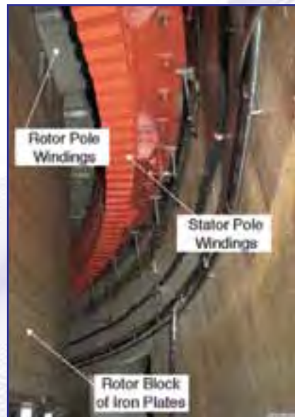
Figure 11: Inside the generator: Stator and rotor pole windings
