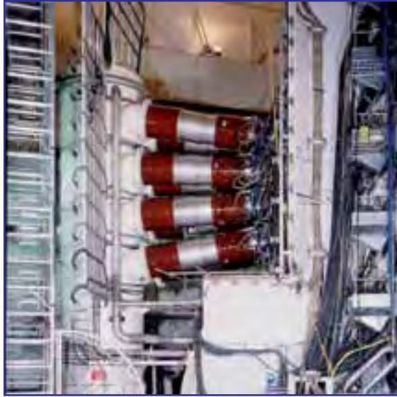
Figure 8: Neutral Beam Injector - JET's most powerful Actuator
