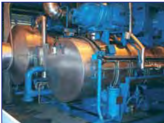
Figure 8: 3 MW chiller unit
