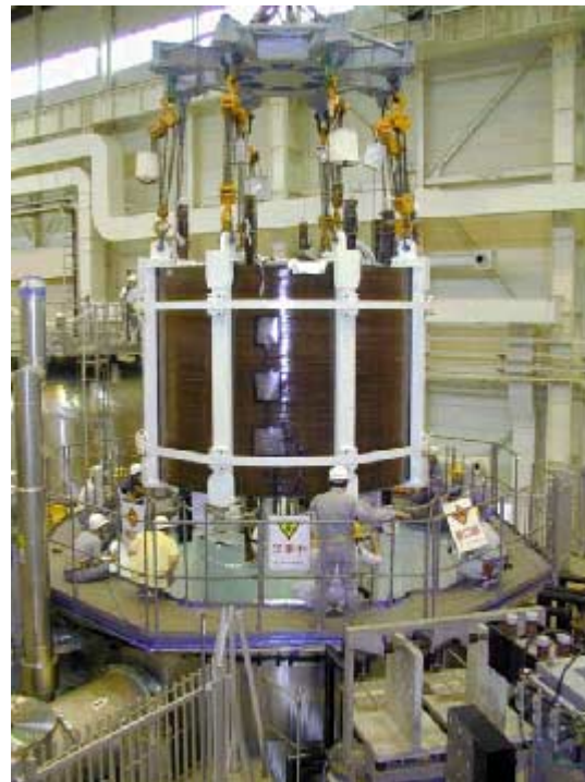
Figure 5.2-1 CS Model coil. The Outer Module being placed outside the Inner Module which has already been installed in the vacuum chamber.
